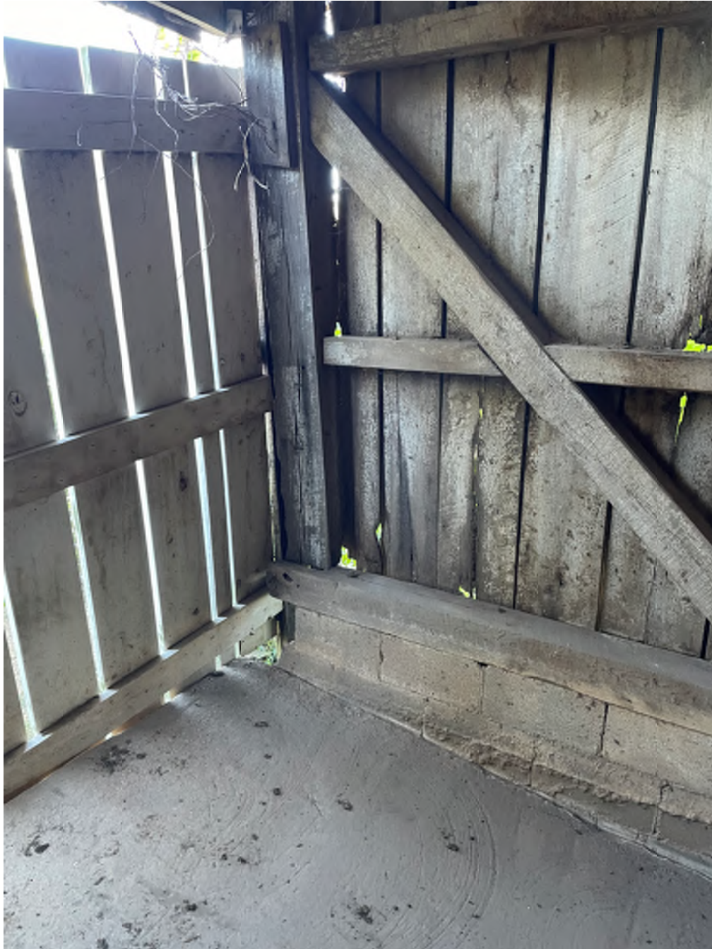
Rotten members at the north west end.
