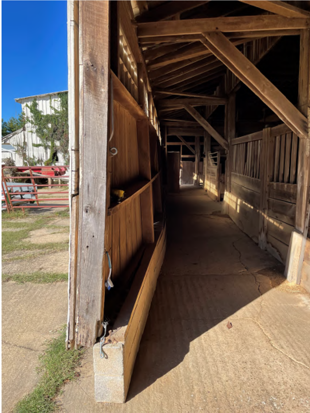
South west foundation wall out of place.
