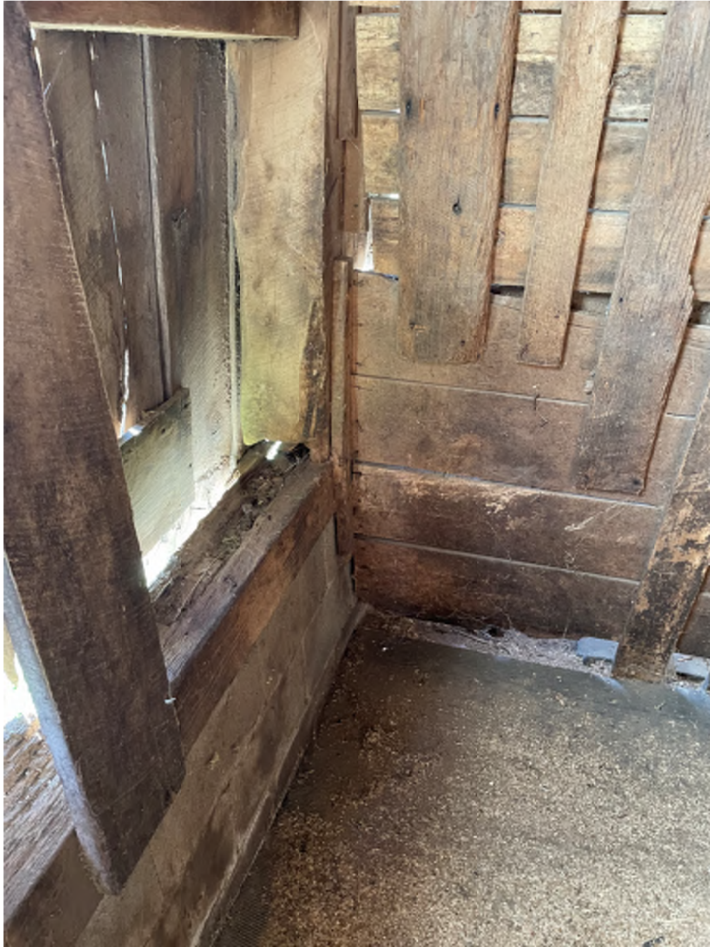
Additional Rotten post.
