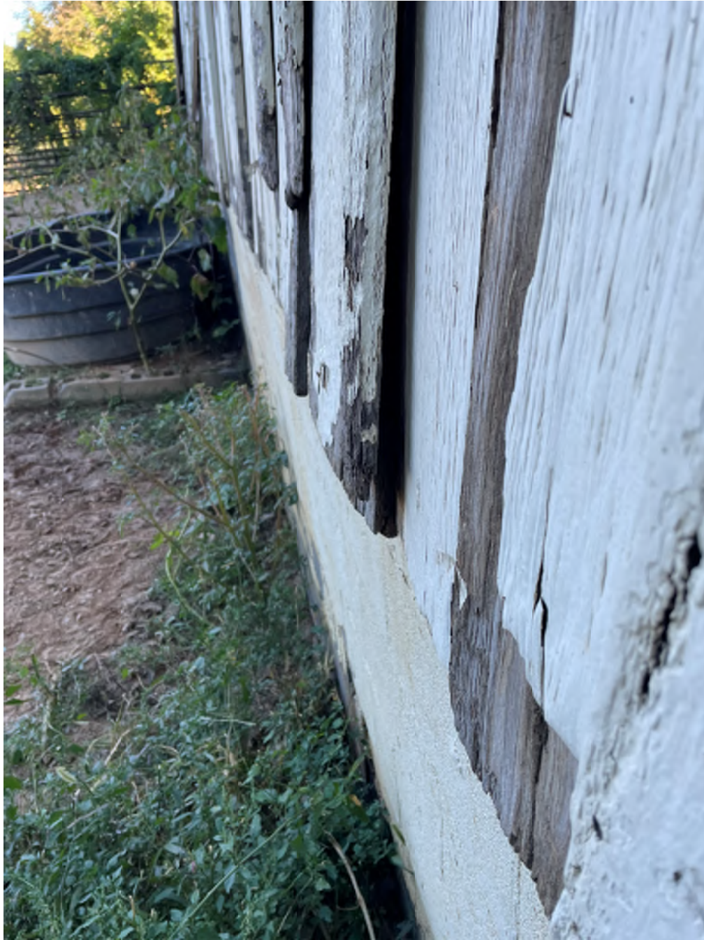
West foundation wall is a retaining wall and leaning outward.
