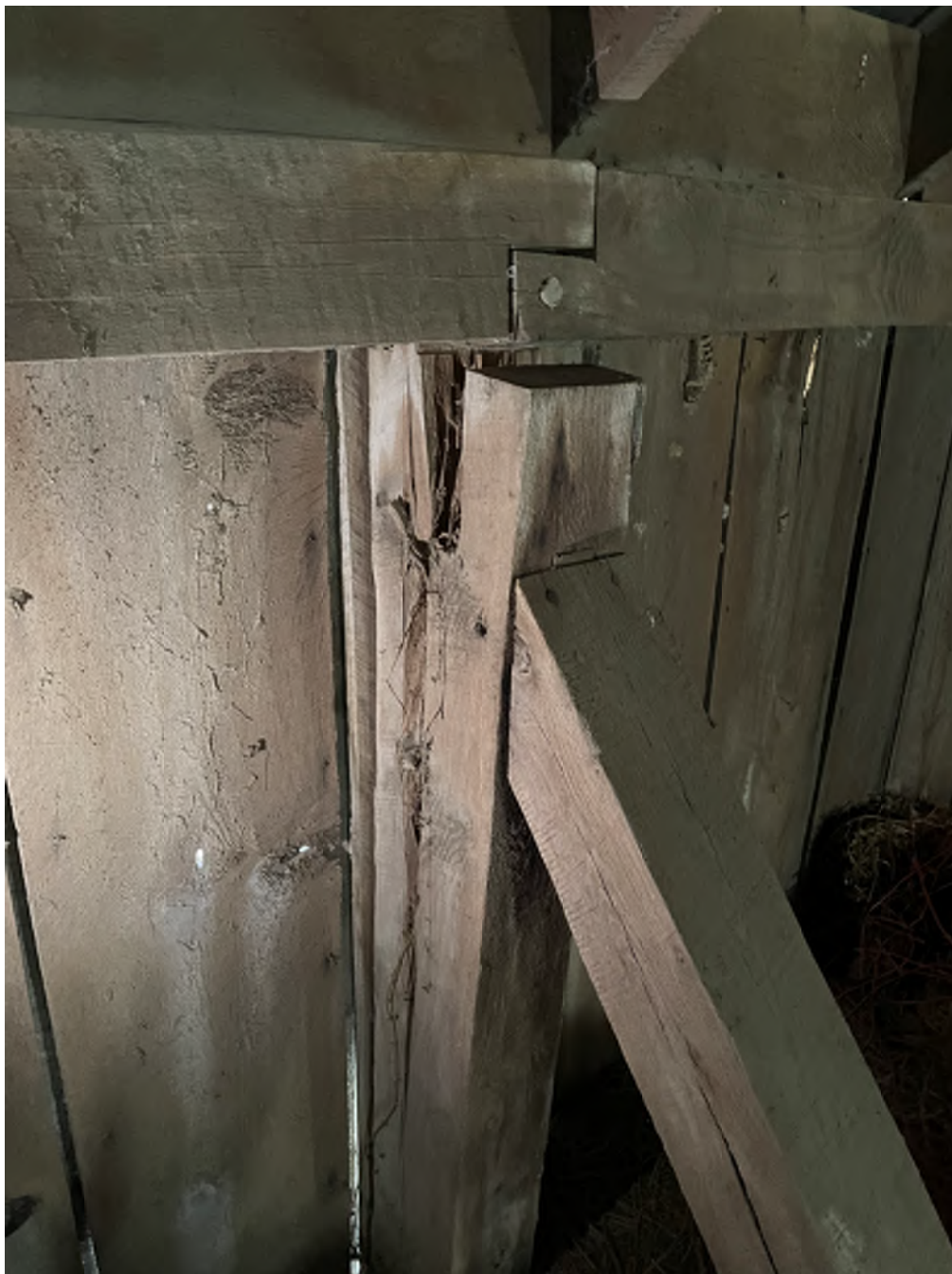
Damaged post in loft
